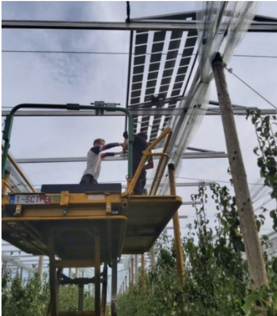
Figure 10: Photograph taken during the installation phase of the agrovoltaic system at Bierbeek.
