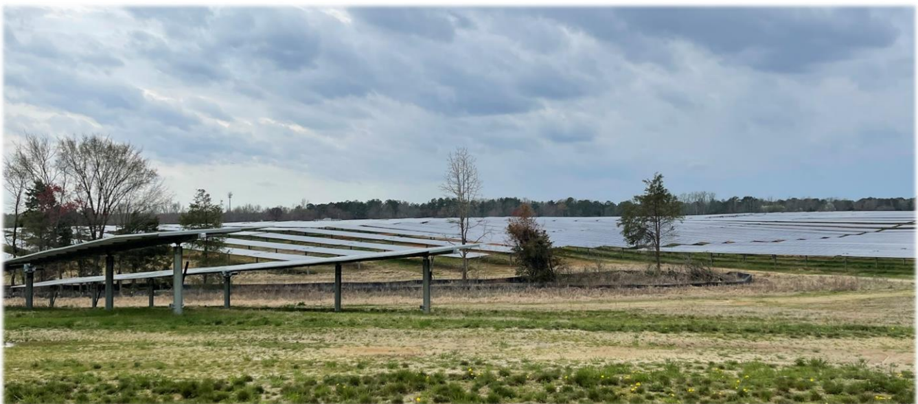
Figure 1. Briel Solar Facility, Henrico County, VA
