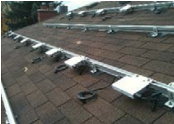
A Solar Electric Racking System
