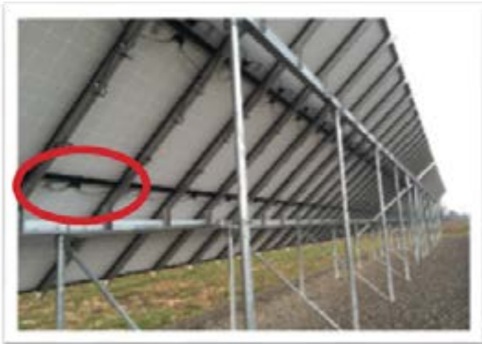
Photo 5 - Conductors over 30V not guarded, installed in raceway, or otherwise inaccessible: NEC 690.31(A)
