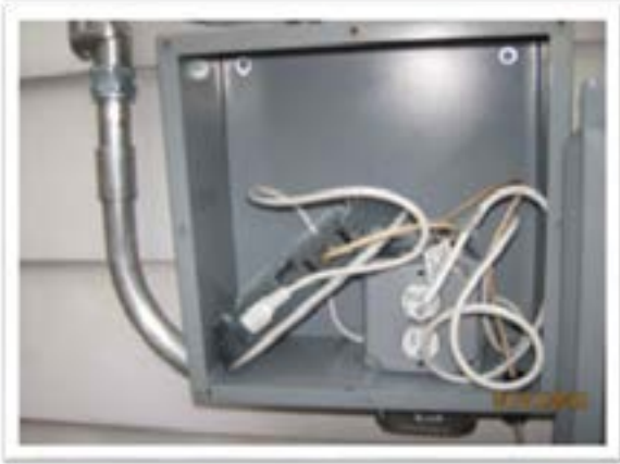
Photo 9: Equipment is not rated for location. In this case, a non-GFCI outlet for PV monitoring equipment is located in a wet location: NEC 110.3(B), 210.8(A)(3)
