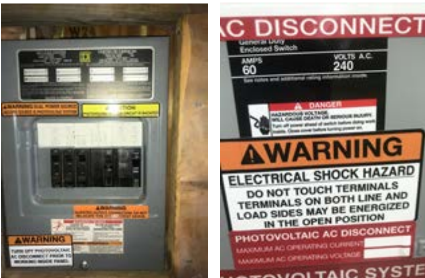
Photo 11: AC disconnect/load center manufacturer's label obscured: NEC 110.21
