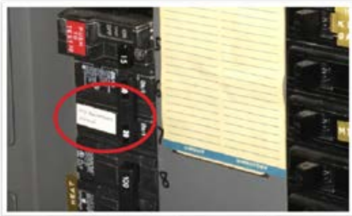
Photo 3: Working clearance not maintained: NEC 110.26
