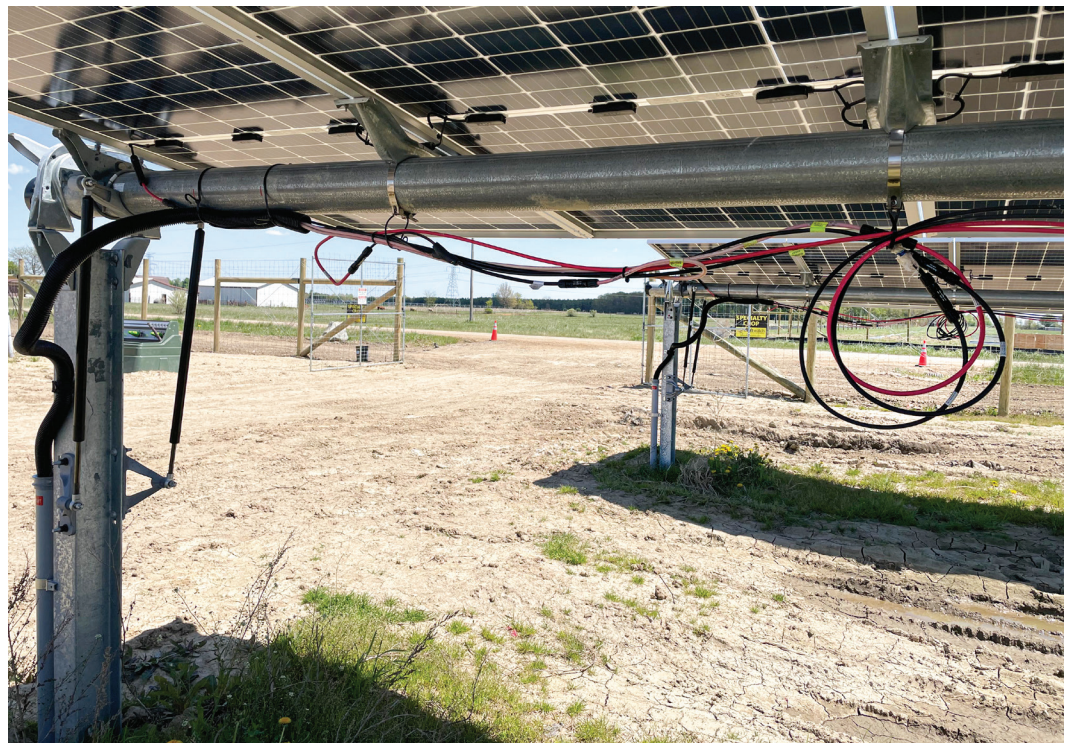
Figure 7. Tray wiring at Assembly Solar in Shiawassee County, Michigan. Cab wiring hangs lower to the ground. (Photo by Sharlissa Moore, May 2021. Adjusted in Adobe Lightroom)
