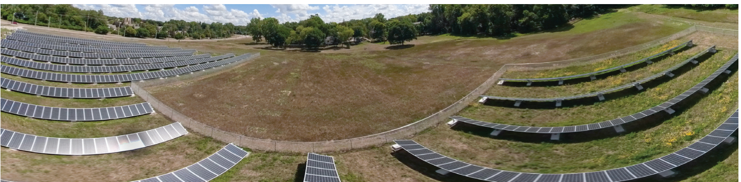
Figure 15. 300 kW solar power plant built on a landfill before pollinator habitat establishment, East Lansing, Michigan. Ballasted system is visible [on the right]. (Photo by Sharlissa Moore, July 2020. Adjusted in Adobe Lightroom)
