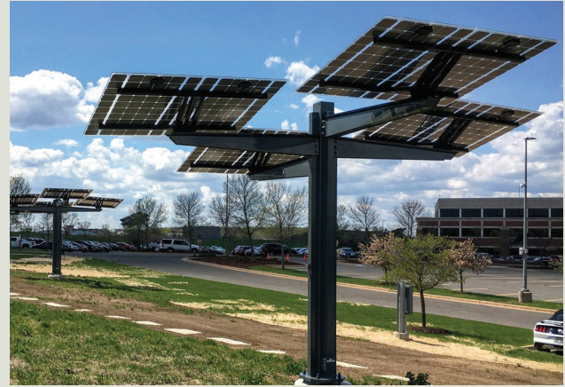
Figure 2: Alliant Energy, Spotlight Solar trees
