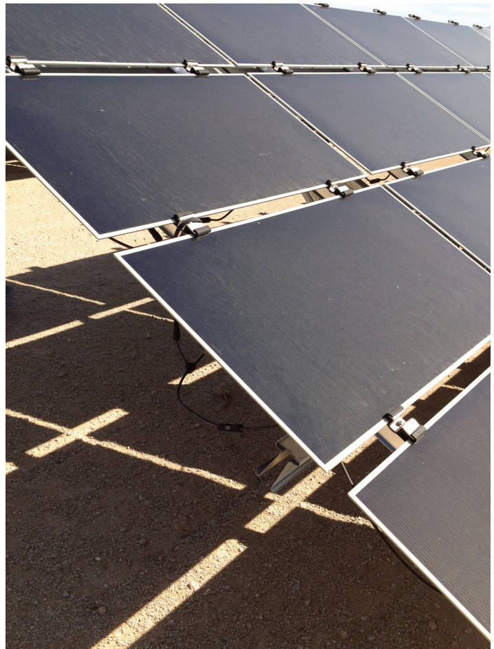
Figure 13. Dust visible on solar modules at a bladed and graded site, Gila Bend, Yuma County, Arizona. APS Paloma Solar Power Plant. The utility company was testing the effect of dust on electricity output. (Photo by Sharlissa Moore, 2014. Adjusted in Adobe Lightroom)
