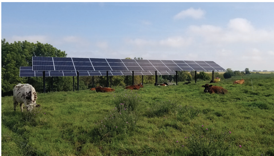
Figure 1. The 30-kW solar photovoltaic ground-mounted system for solar shading at the University of Minnesota West Central Research and Outreach Center in Morris, Minnesota.
