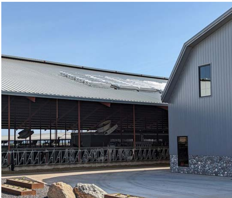
Winston Cone Optics Solar Thermal System. Photo: Winston Cone Optics
