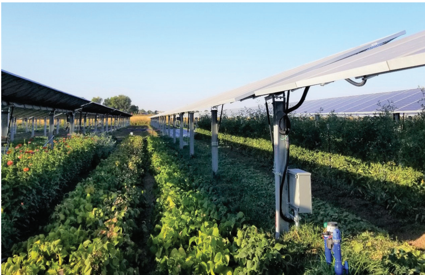
Single-axis tracking system at Jack's Solar Garden. Photo: AgriSolar Clearinghouse
