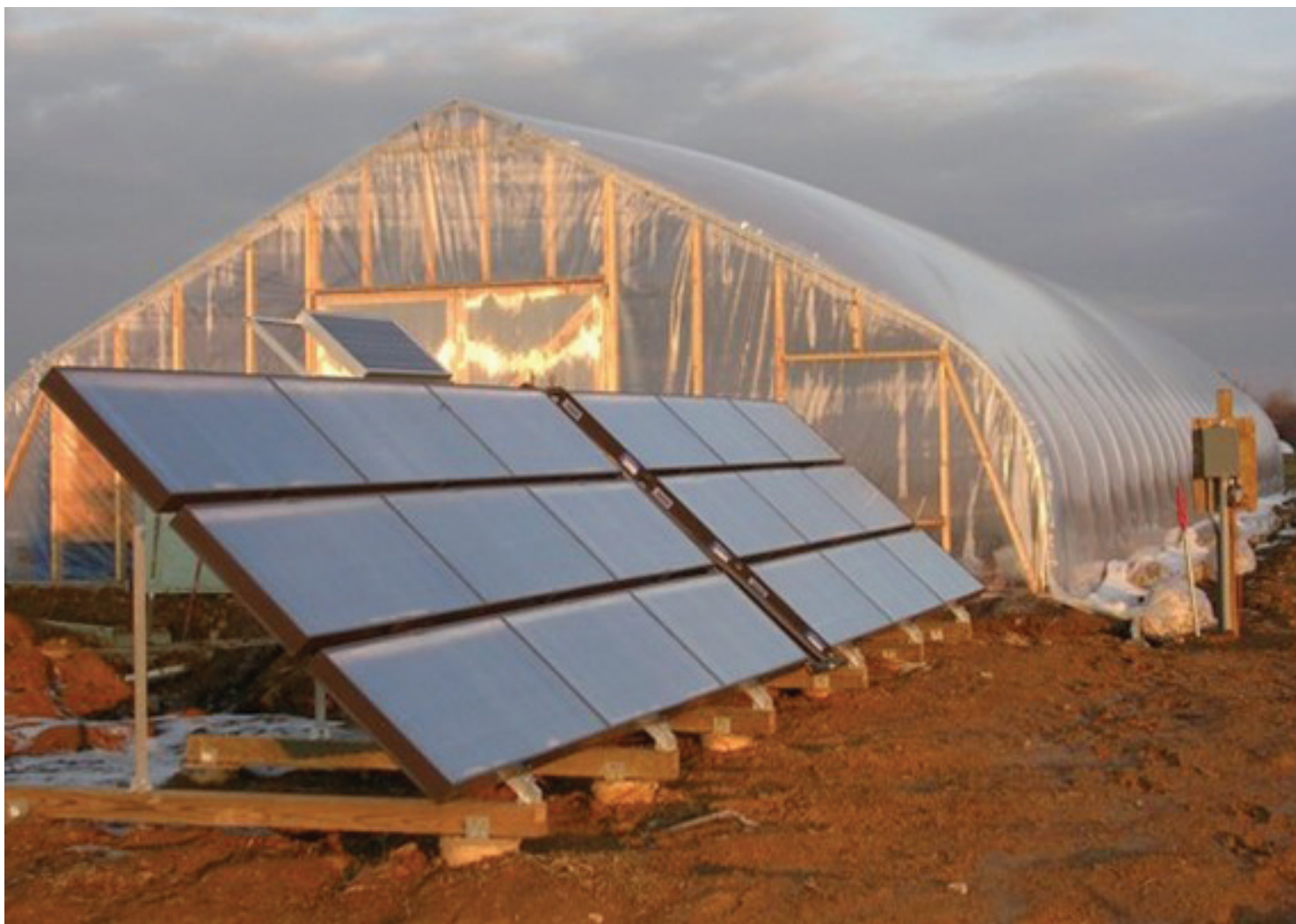
Solar thermal flat-plate collectors heating a high tunnel. Photo: AgriSolar Clearinghouse
