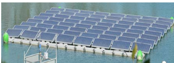
Fig. 9. 14kWp Floating System in Piolenc, France [21]
