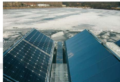
Fig. 10. 20kWp FTCC System in Cheogji, South Korea with can withstand water freezing temperatures [24]
