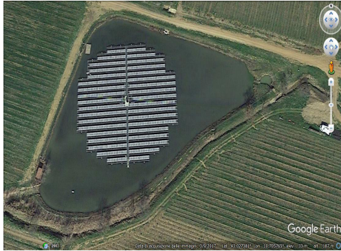
Figure 1. The PVF plant with tracking on the Suvereto (Italy) irrigation basin
