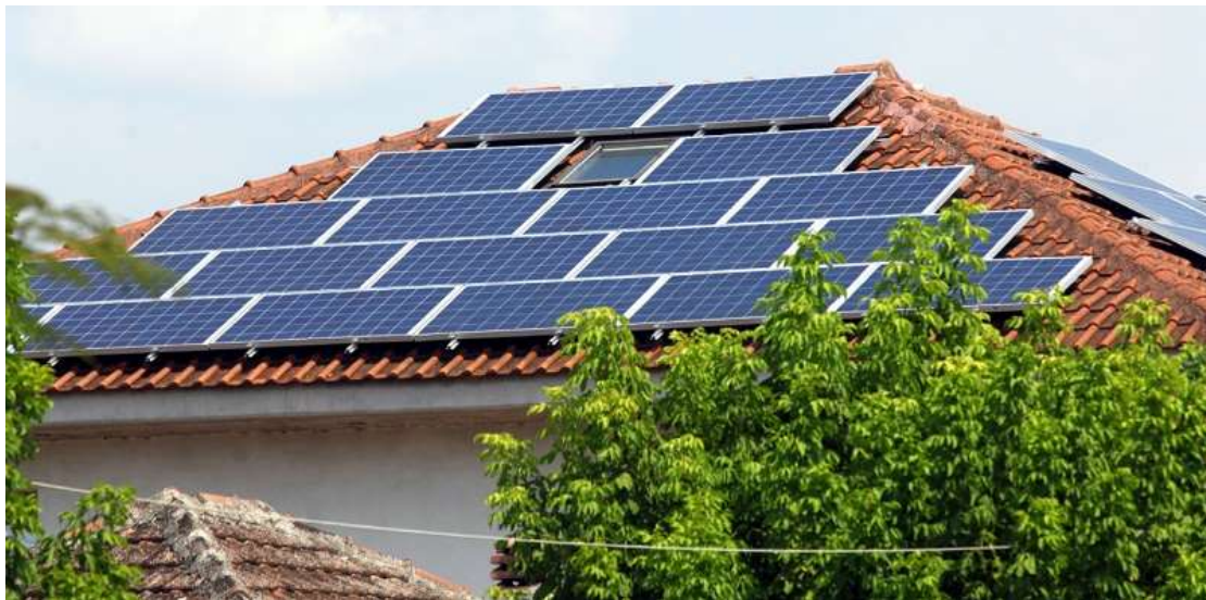
Figure 22. Typical domestic solar array, Greece
