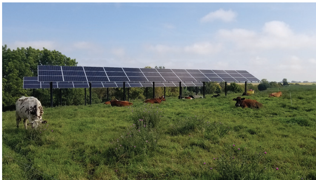
Figure 1. The 30-kW solar photovoltaic ground-mounted system for solar shading at the University of Minnesota West Central Research and Outreach Center in Morris, Minnesota.
