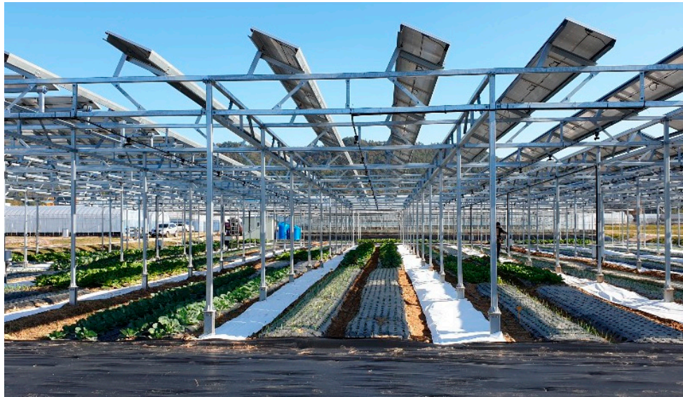
Figure 1. Farm-type photovoltaic-power-generation system.
