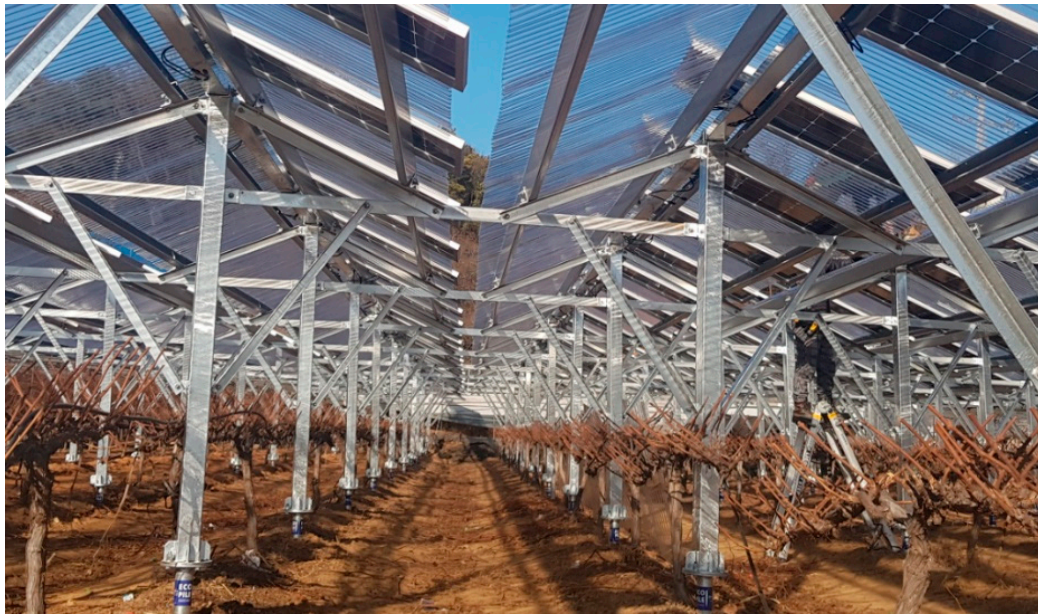
Figure 3. Rain-hit-protection solar facility in a grape farm.
