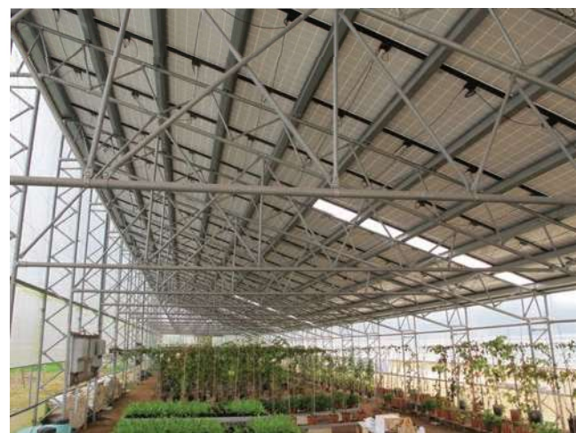
Figure 2. Tested photovoltaic greenhouse at experimental field of Avetrana (Taranto), internal view from Western gable wall.
