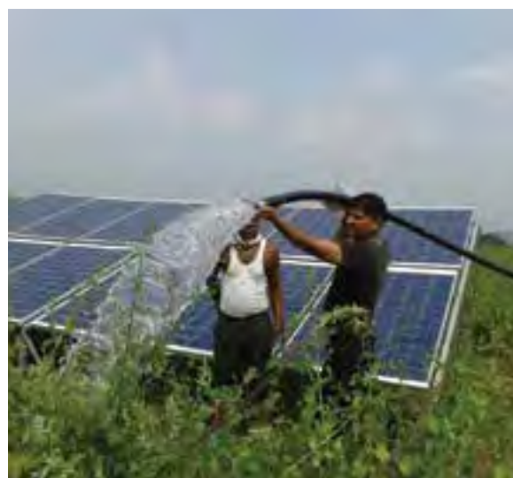
Solar water pump in India
