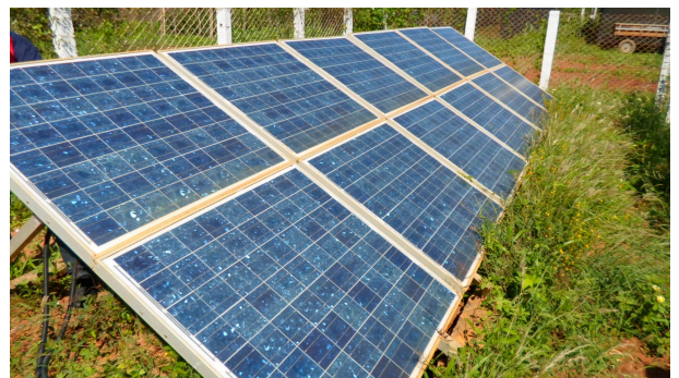
Fig. 6. Microgeneration installed at UEPE. Source: Author.
