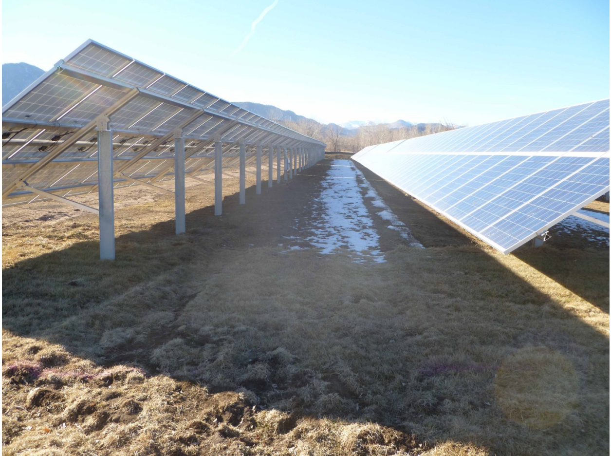
Photograph 11. Fixed panel photovoltaic array at University of Colorado East Campus, arranged in east-west rows, maximizing shading effects. View faces west. Photo Credit: Dave Buckner
