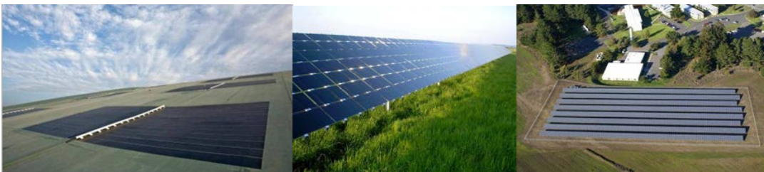
Figure 4. Thin-film solar panels installed on (left) solar energy cover and (middle, right) fixed-tilt mounting system. Photos by (left) Republic Services, NREL 23817, (middle) Beck Energy, NREL 14726, and (right) U.S. Coast Guard Petaluma Site, NREL 17395
