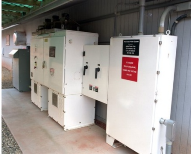
Figure 5. String inverter. Photo by Warren Gretz, NREL 07985
