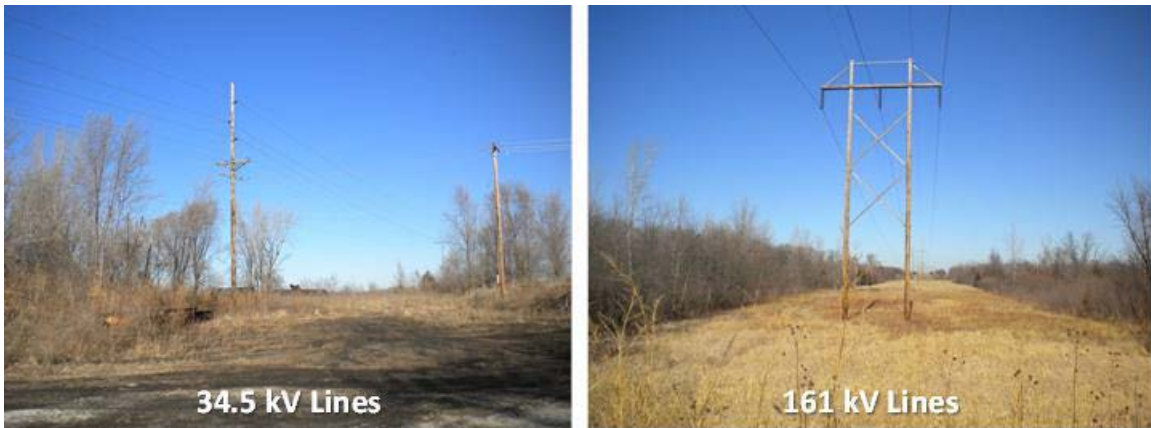
Figure 8. Electrical transmission lines for the PV system at the site. Photos by Jimmy Salasovich, NREL
