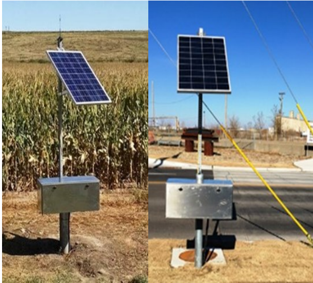
Solar-powered traffic counters in Dodge City, KS (left) and Topeka, KS (right). Source: Kansas DOT
