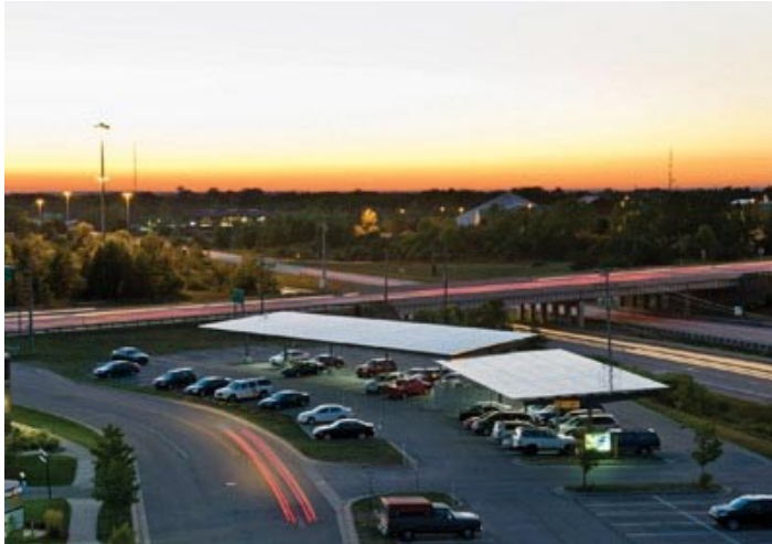
MDOT installed two solar-powered carports at a parking lot at the interchange of State Route 44 and I-96 in Grand Rapids, MI. Electricity generated by the array powers the lighting at the interchange. Source: Michigan DOT Photo Lab
