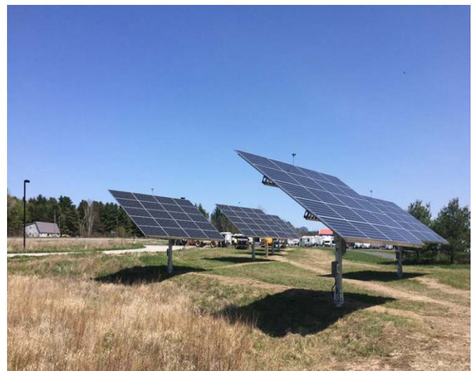
Figure 3: Solar panels at the Fair Haven, Vermont Welcome Center (Source: VTrans)
