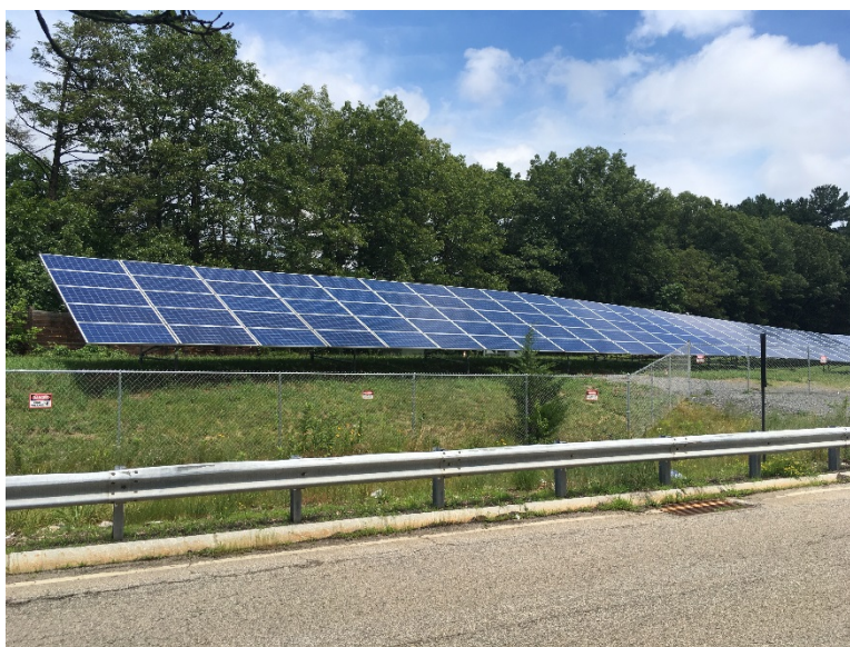
Figure 1: Solar panels at the Framingham Service Plaza on Interstate 90 (Source: Volpe Center)
