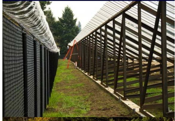
Installation of the steel racking system, aluminum framing and solar PV modules.
