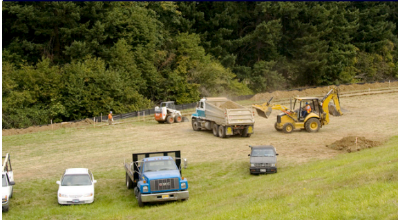
Site preparation including grading and construction of the solar PV array footings.
