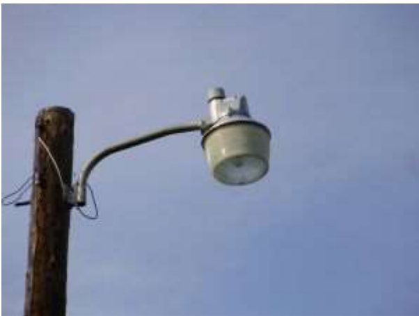
Mercury vapor yard light. Photo credit: Carl Pederson
