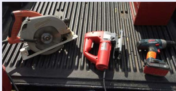
A circular saw, a jig saw, and a screw gun are the only power tools needed for the installation. Photo: Chris Lent, NCAT
