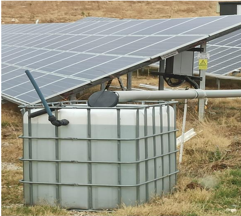
Fig. 6. First attempt for rainwater harvesting with 1 m 3 tank.
