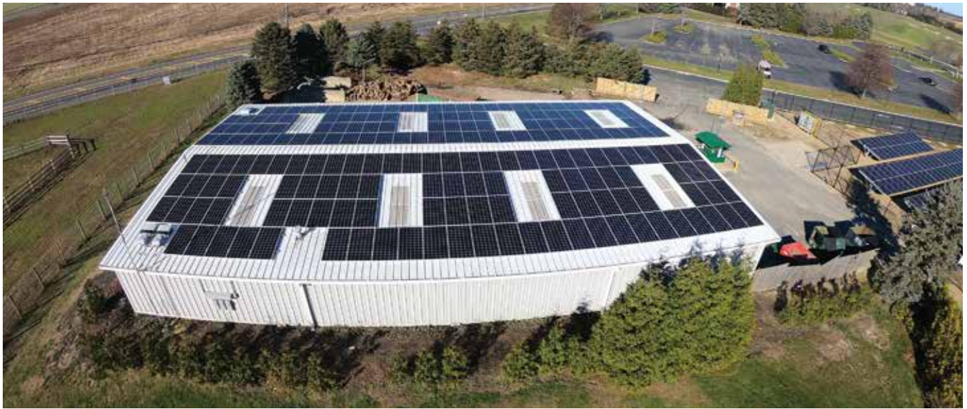
Rooftop and ground-mounted solar arrays at the Long Island National Golf Club in Riverhead © SUNation Solar Systems
