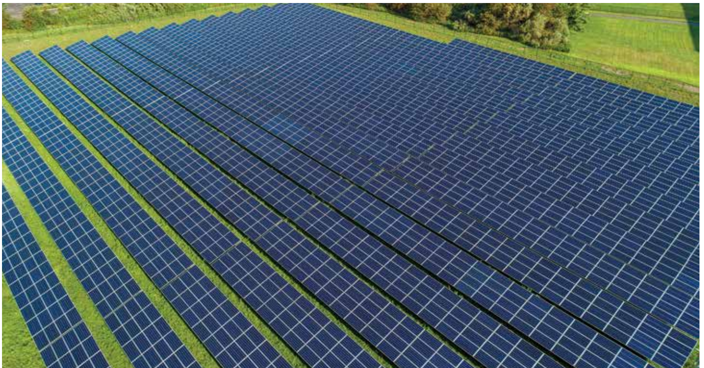
Ground-mounted solar at the Estee Lauder Companies’ campus in Melville, NY. © EmPower Solar
